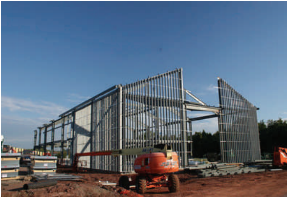
Structural components of the new worship center have now been put in place.
